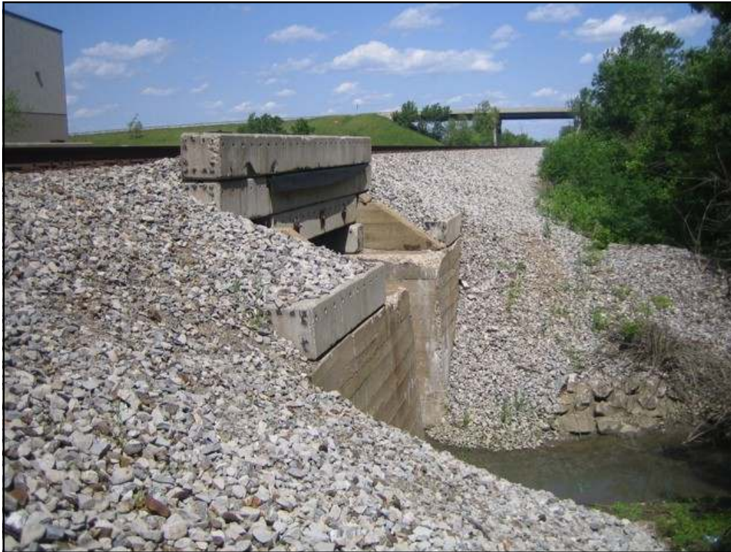
This photo shows the vulnerable south side of the Lakeside development, incorporating the Norfolk-Southern railroad tracks as flood protection. These holes must now be filled permanently.
